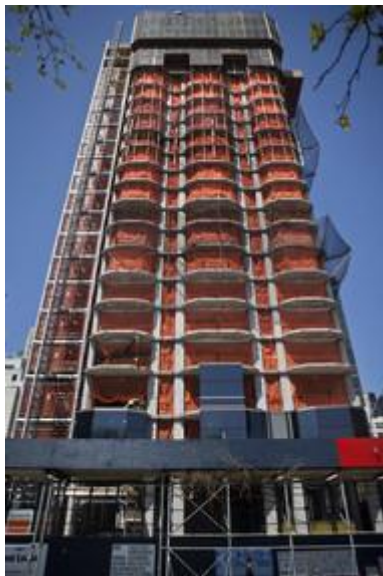
The 50 UN Plaza building stands under construction in New York during April 2013. Photographer: Victor J. Blue/Bloomberg
